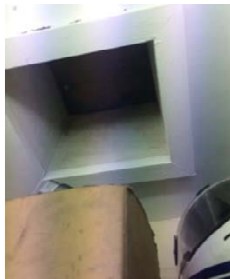
Photo 2 - Water stained old roof light box
