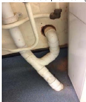
Photo 5 - Poor finish to plumbing
