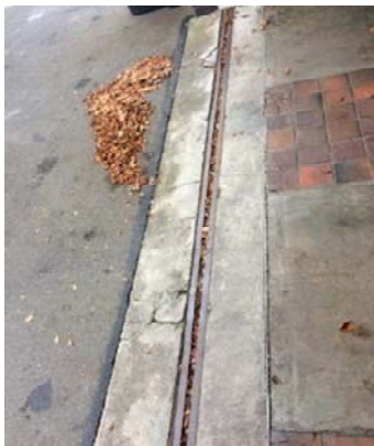
Photo 1 - Cracked concrete ramp
