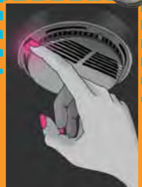
No battery in the smoke alarm
