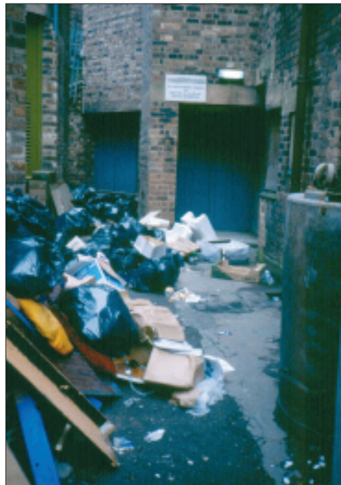
Figure 9: A blocked escape route (courtesy of the Association of British Theatre Technicians)
