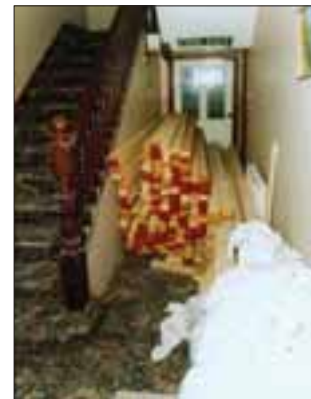
Figure 9: A blocked corridor with incorrect signage
