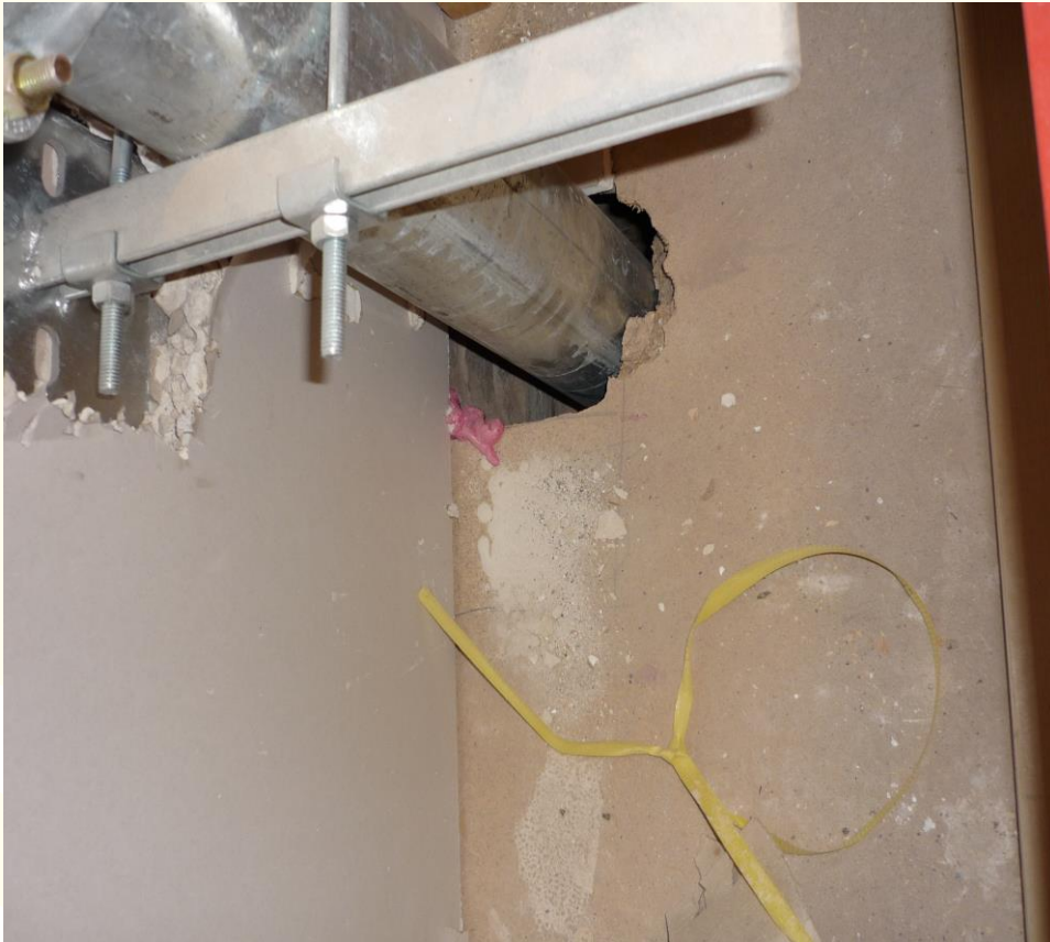
No Fire Stopping
